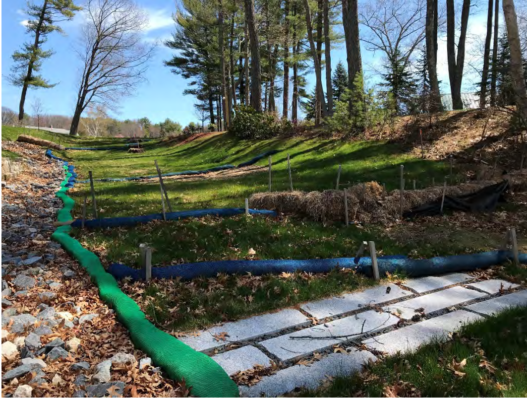
Fig 9: Slope above the manhole at Gundalow Landing/east side of the bay. Viewing east. (04-19-21)
