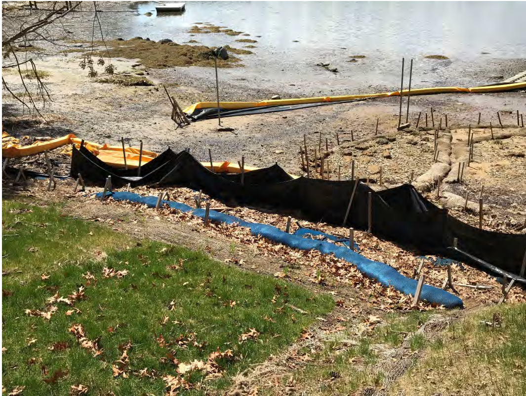
Fig 11: Toe of the slope at Gundalow Landing/east side of the bay. Viewing south. (04-19-21)
