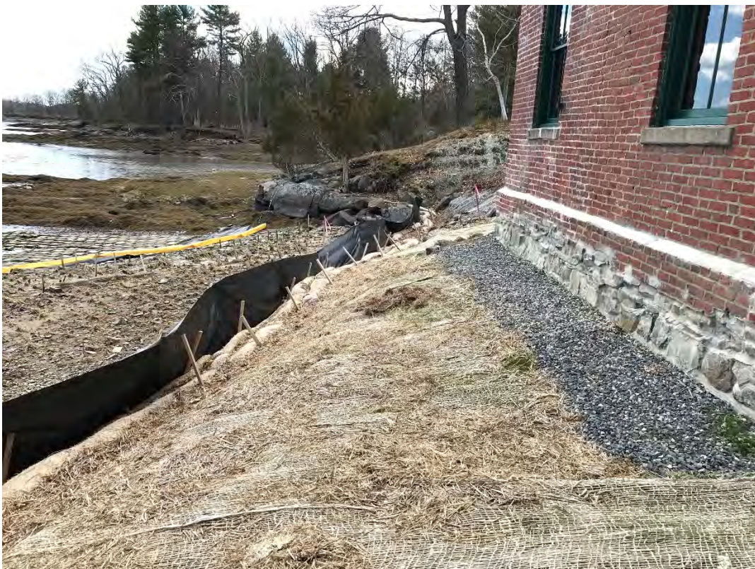
Fig 2: Slope between the cable house and salt marsh restoration at the west side of the bay. Viewing south. (04-19-21)
